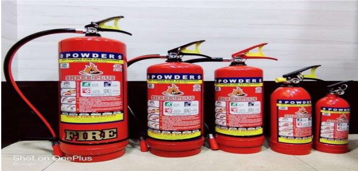
Fire extinguishers available in whole campus
