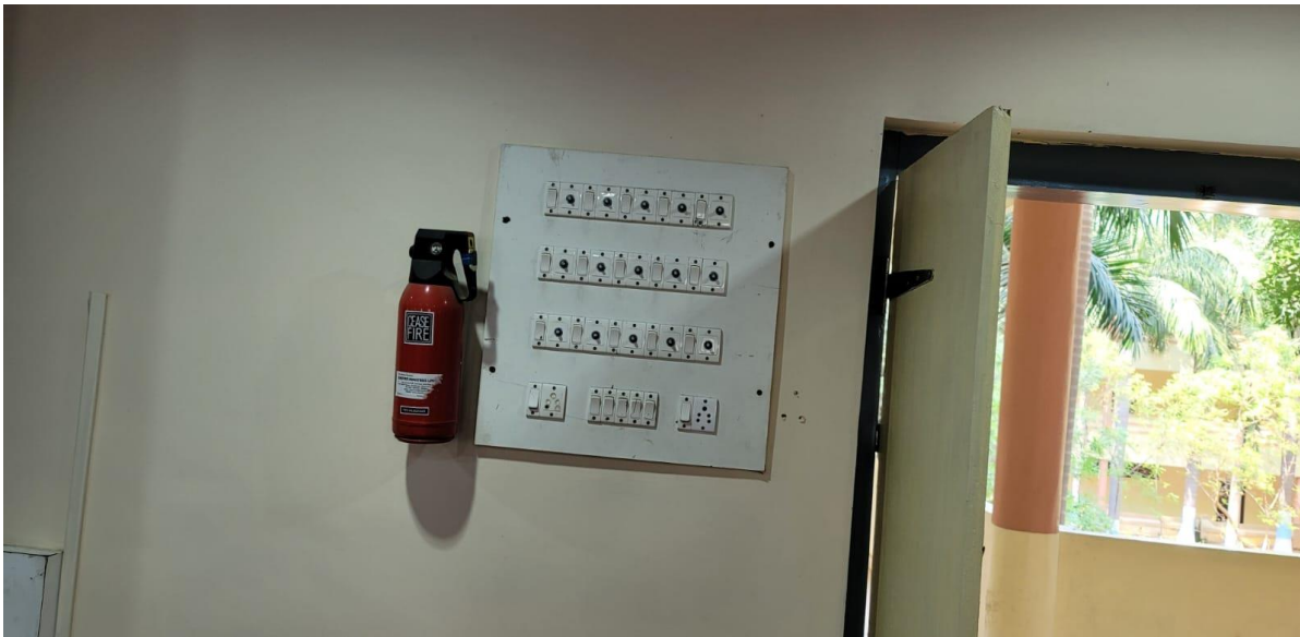
Fire extinguishers available in whole campus
